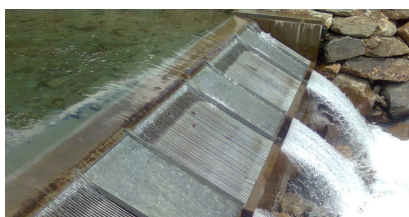
(a) River installation (www.guflermetall.it)
